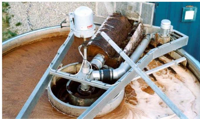
Plate 2.6: The main DAF treatment tank at Arpley Landfill
