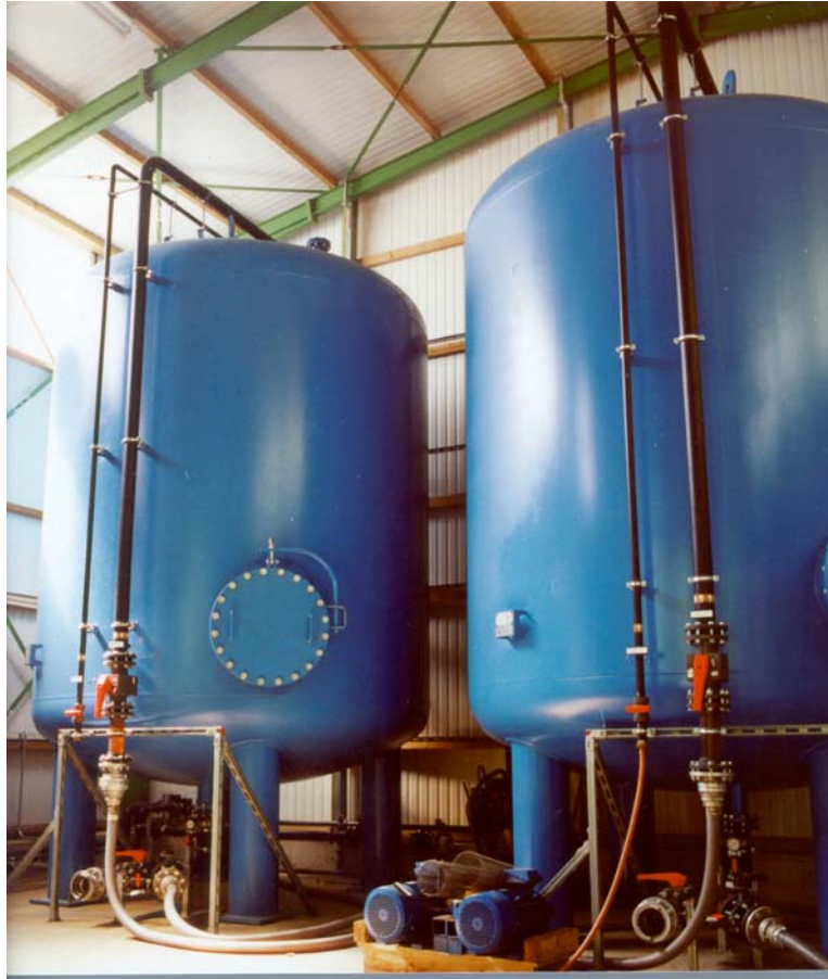
Plate 2.8: Typical internal sequential GAC tank installation for polishing of biologically-pre-treated landfill leachate
