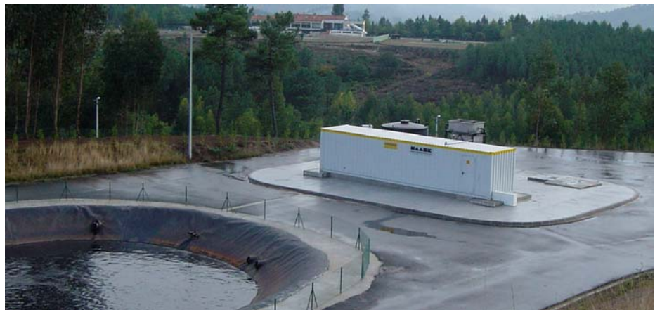
Plate 2.5: Typical configuration of a 2-stage RO plant with aerated leachate lagoon, direct permeate discharge and concentrate re-infiltration (120 m 3 /d, Rebat landfill, district of Amarante, Portugal, commissioned 2001) (see Loeblich 2005)
