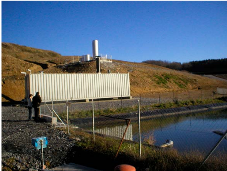
Plate 2.3: Typical configuration of a 2-stage RO plant with leachate lagoon, direct permeate discharge and concentrate re-infiltration (72 m 3 /d, landfill CSDU Pays des Graves, district Hautes-Pyrenees, Commune de Lourdes, France, commissioned 2004) (see Wachter 2005)
