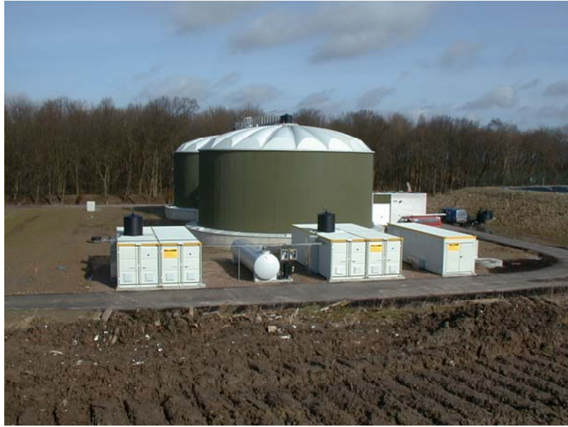
Plate 2.2: Typical configuration of two 2-stage RO plant with leachate tanks, direct permeate discharge and concentrate re-infiltration (350 m 3 /d, Niemark landfill, Luebeck Germany, commissioned 1999).
