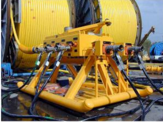
Umbilical attached to umbilical termination assembly
