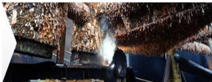
Typical marine growth contamination found on jackets
